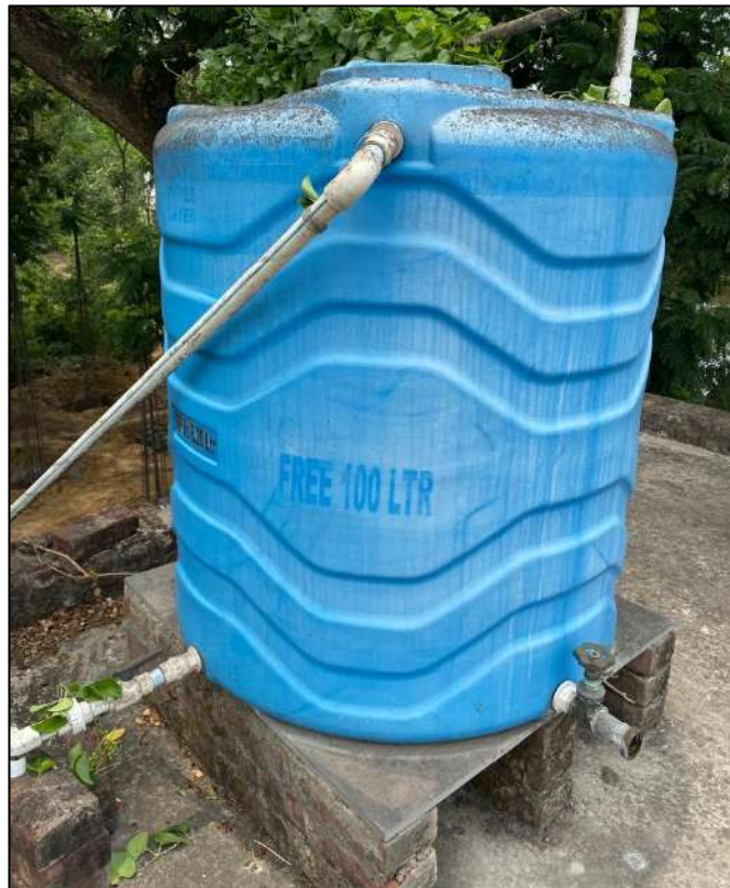
Tank on the roof of Bio-Science Building
