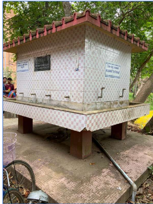
Drinking water reservoir and connected pipeline
